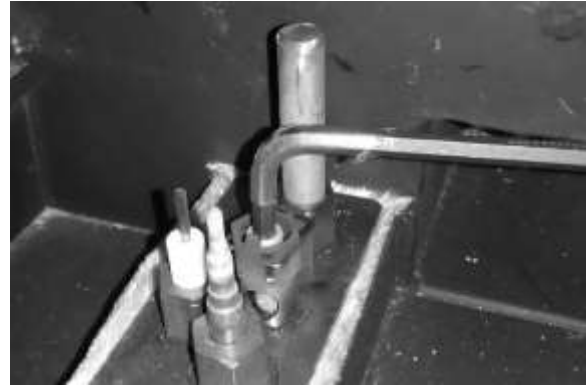
Figure 8 – Loosening Pilot Orifice
