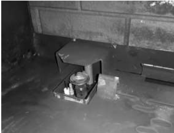
Figure 11 – Pilot, Shield, and Burner Position
