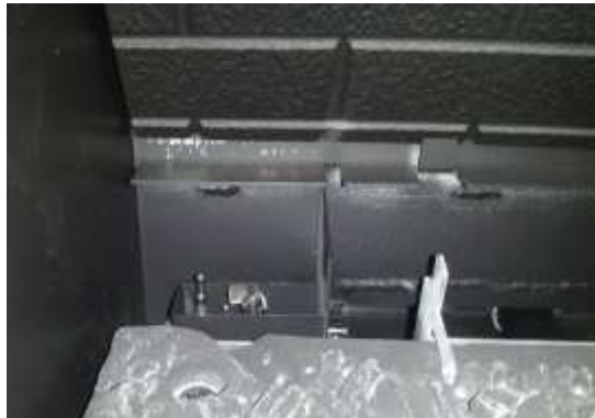
Figure 6 – Pilot, Shield, and Burner Position
