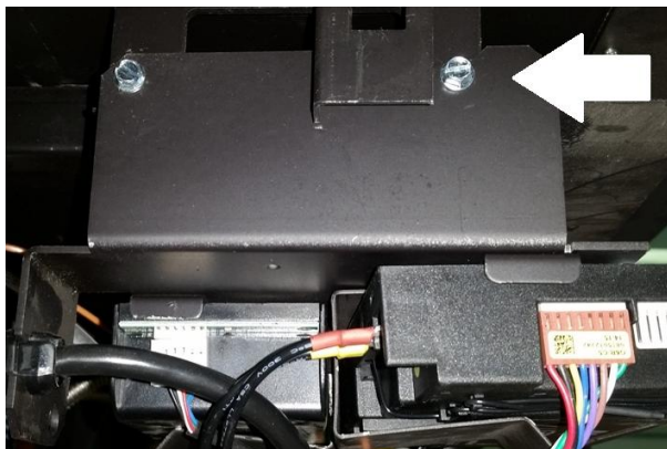
Figure 4 – Front Valve Mounting Bracket Screw (from left side of stove)
