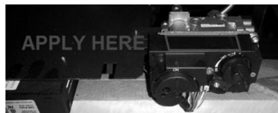
Figure 15 – Valve Warning Label Location
