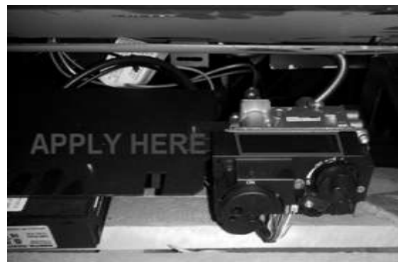
Figure 17 – Valve Warning Label Location
