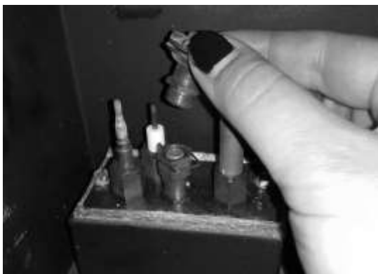
Figure 7 – Removing Pilot Burner Hood
