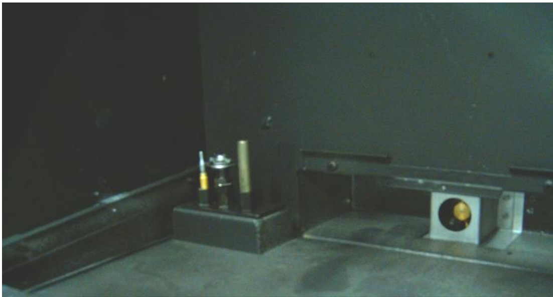
Photo #4 Pilot assembly (left) and air shutter with burner orifice (right) in the firebox after the pan burner is removed
